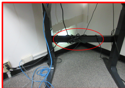
2. Wrapping the power cord around the fixed crossbar at base or hung up on stationary elements, e.g., under table foot or CPU
