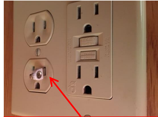
Broken Blade in “Hot” side of outlet SERIOUS SHOCK HAZARD!
