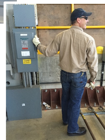
480V, 60A Disconnect Switch, All Covers in Place
