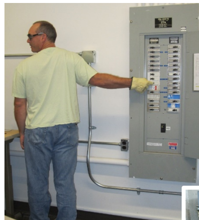
208V Panel, 225A Main, All Covers in Place
